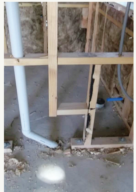
Another bad job with an unreinforced cut-out in the wall framing.
