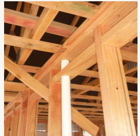
What not to do – unreinforced cut-out in timber framing.
