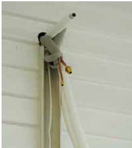
a. Hoses coming through the top of the exterior wall.
