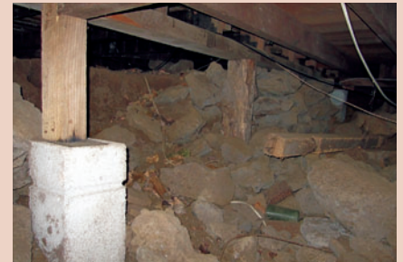
Figure 3: Today's restored Alberton (originally built 1863) with a modern timber jack stud in the foreground on top of a pre-cast concrete pile and the original timber pile with scoria wall behind.
