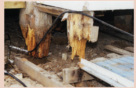
Figure 2: 90-year-old totara piles after house lifted (hydraulic pipes connecting the central pump to distributed lifting jacks are visible).
