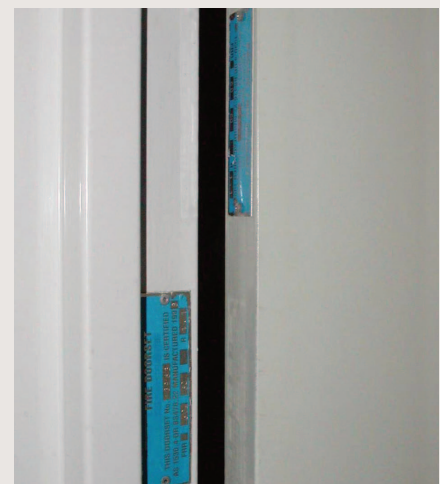
Figure 4: Fire door tag attached to the leaf and the door frame.
