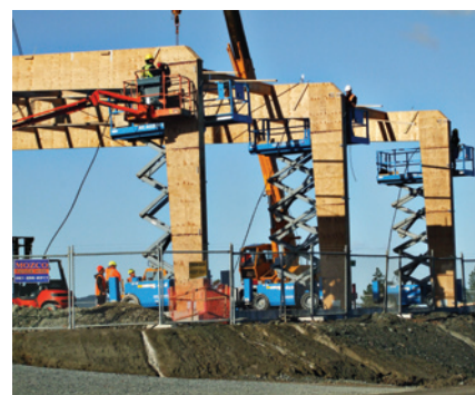
Laminated veneer lumber roof lift at Whangarei mill. (Photo: Carter Holt Harvey.)
